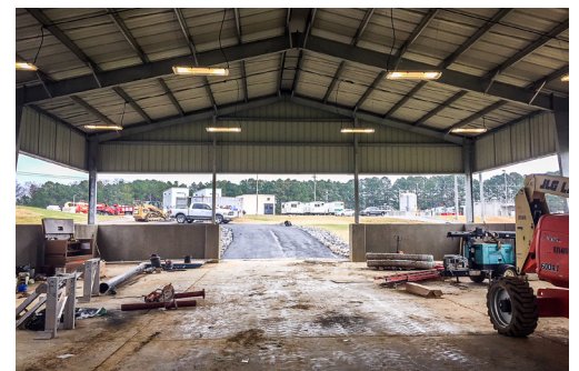
The covered sludge pad is designed to store sludge for a 60-day period while also providing a storage site for equipment
