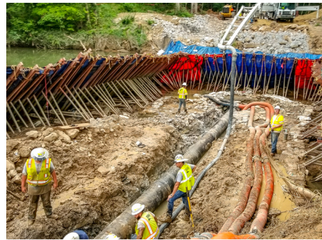
Temporary dams were constructed at each site where the waterline had to cross the South Chickamauga Creek.
