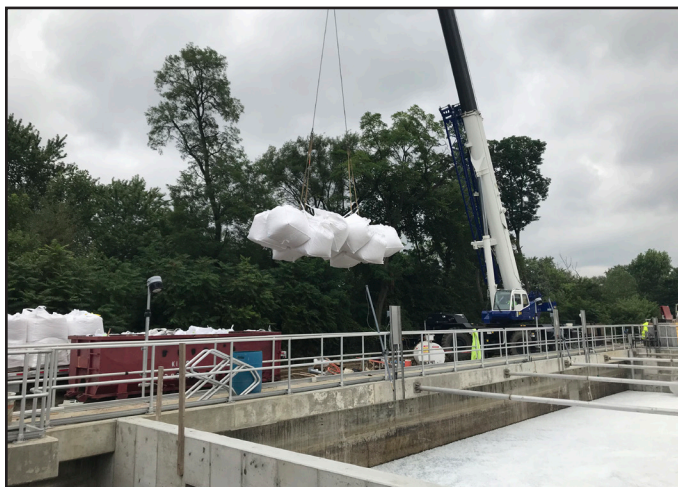
Bags containing IFAS media being placed in the oxic zone of the aeration tanks
