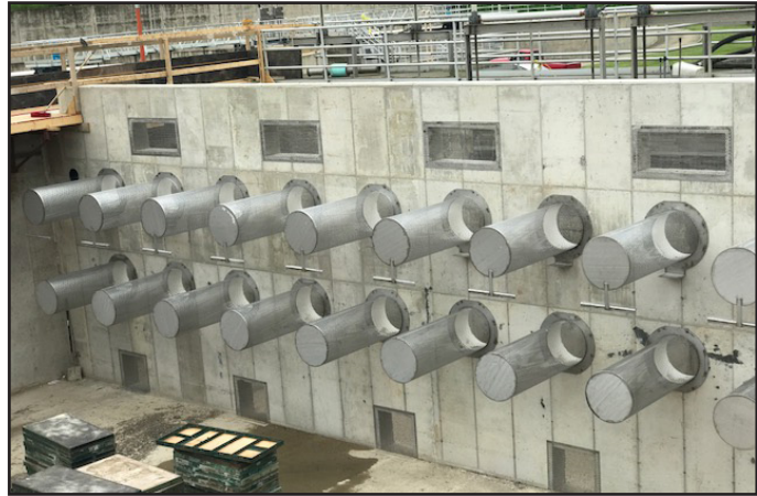
Cylindrical effluent screens at the end of the aeration tanks during construction
